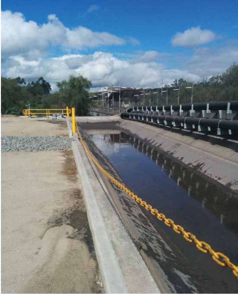
Figure 34: The completed sediment basin on the north-east side of the Hunter River Bridge
